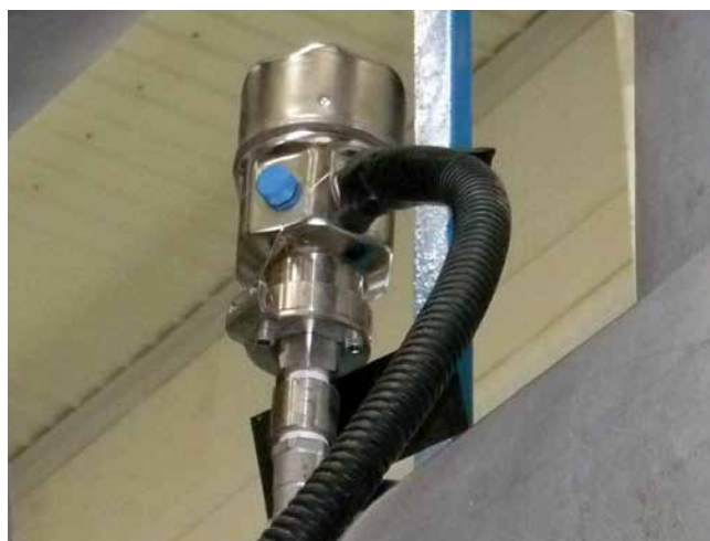
Reliable pressure measurement in a membrane system
