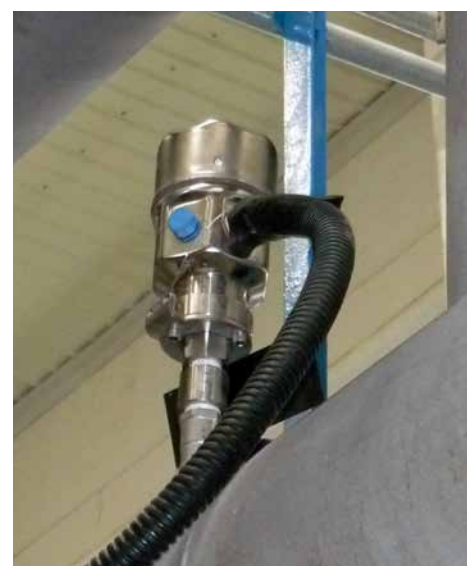
Accurate pressure measurement in a membrane system
