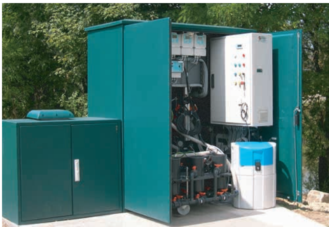
Compact water body monitoring station with container solution
