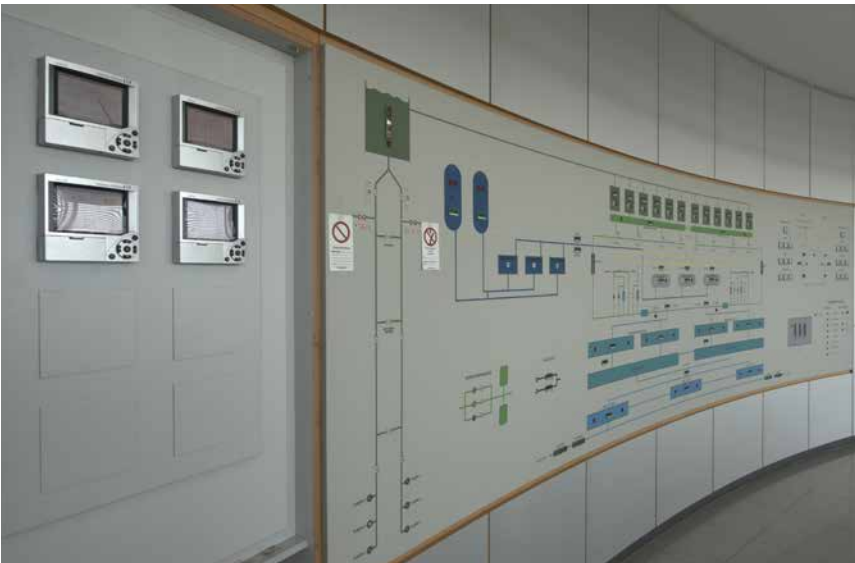
Always on: Data loggers and indicators for cabinet and control center
